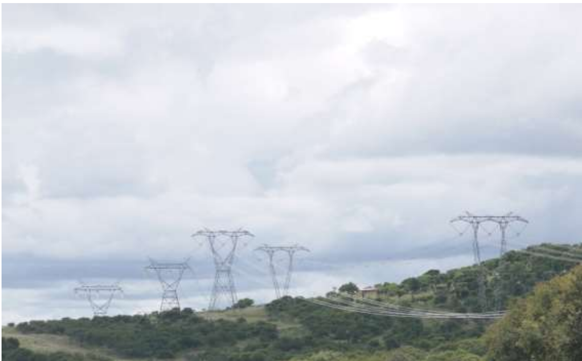
Plate 12 - Existing 400kV double overhead transmission lines are highly obvious as they cross ridgelines from short distance (approximately 1km).
