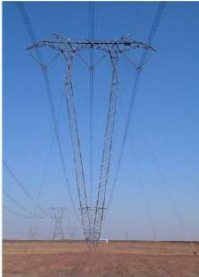
Figure A-5: Tower Type 520B (Guyed V).
