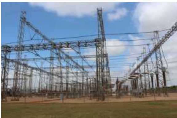
Plate 5 - Sub-station Bus Bars
