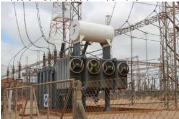
Plate 7 - Transformer showing oil reservoir and fans for cooling.
